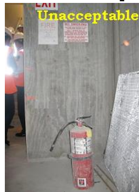
Improper floor placement of Fire Extinguisher.
